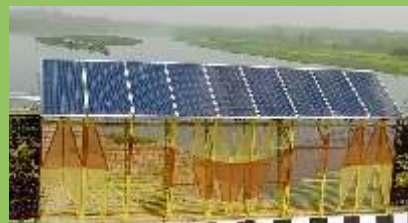
Electrification through Solar Power of 1050 kWp
