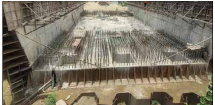
Fig.16 Visible Dowels Left in the Bottom Slab and Walls along with Pockets Left in Bottom Slab for Piling after Box Pushing
