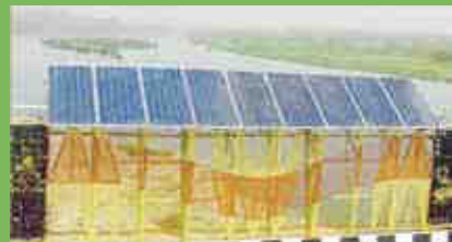
Electrification through Solar Power of 1050 kWp
